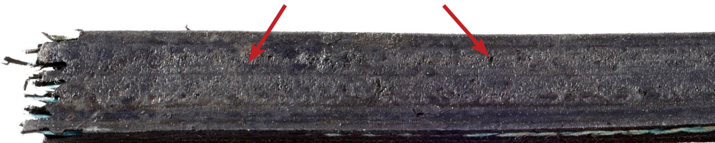
Evidence of overheating caused by compressor slugging.
